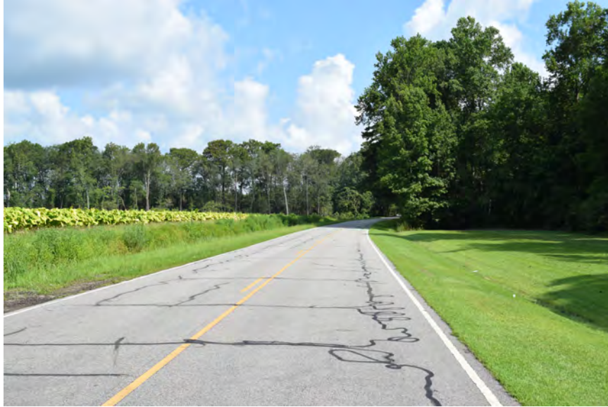
Market Street Extension (SR 1422) in front of the Agnes and Wiley S. Woolard House, view to the north toward Bridge No. 6
